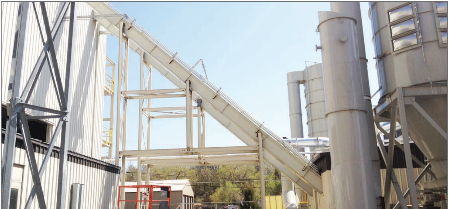
The redesigned L Path En-Masse Conveyor System effectively handled feedstock from truck unload to the storage silos.
